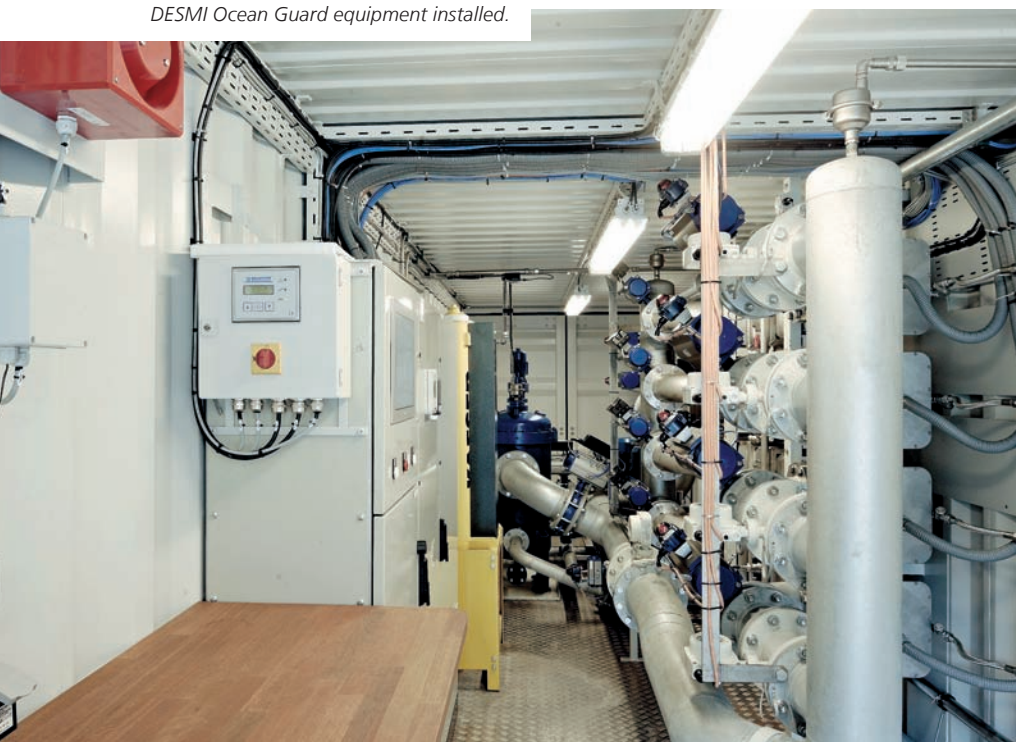
DESMI Ocean Guard equipment installed.
